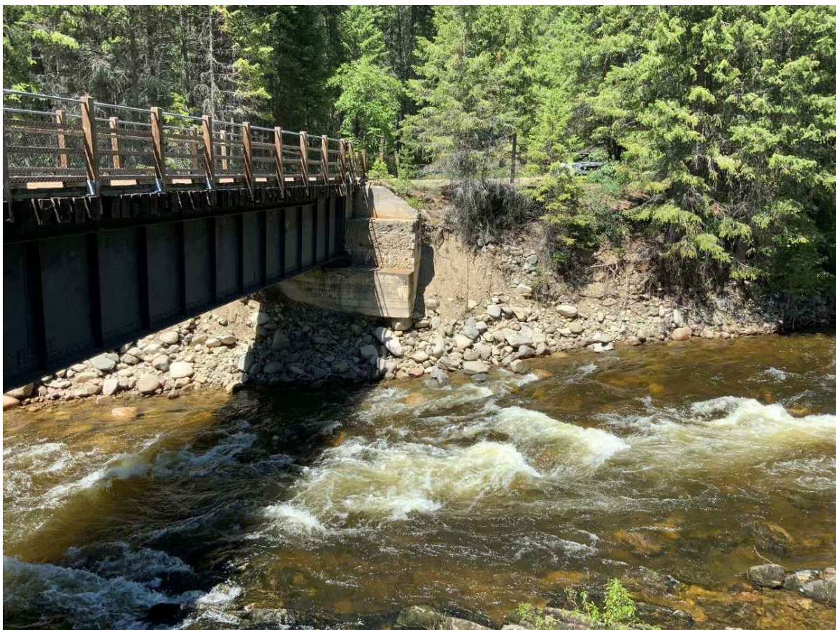
PHOTO 6: EROSION AT THE "RIGHT" BANK UPSTREAM OF BRIDGE
