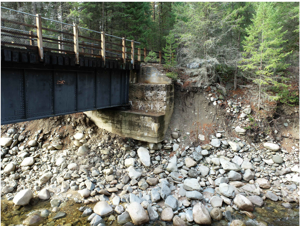
PHOTO 3: EROSION AT THE "RIGHT" BANK AND UNDERMINING AT THE ABUTMENT ON THE UPSTREAM SIDE OF BRIDGE
