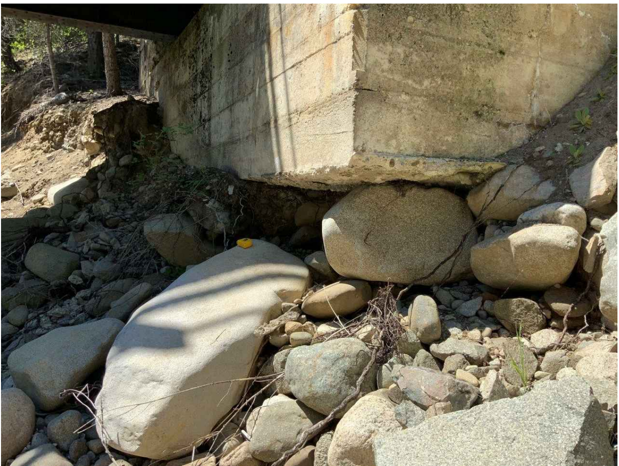
PHOTO 4: UNDERMINING AT THE "RIGHT" ABUTMENT
