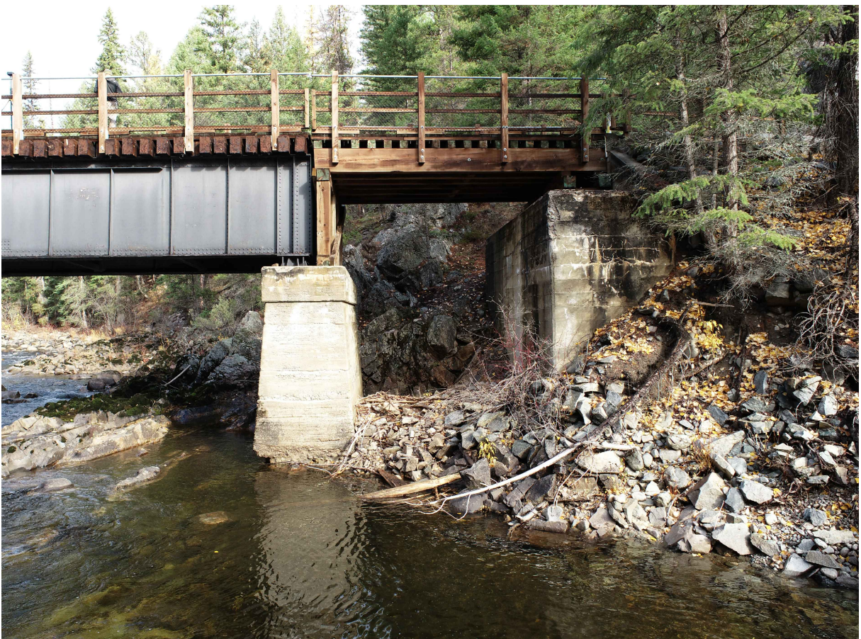
PHOTO 8: UNDERMINING AT THE DOWNSTREAM CORNER OF PIER
